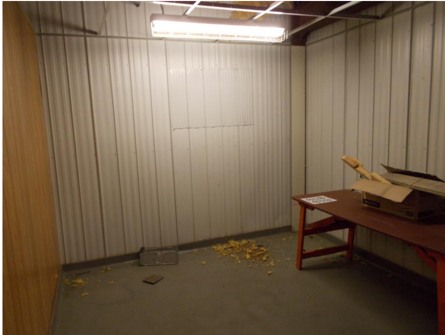
PHOTOGRAPH 7: Showing interior building materials, also showing insulation observed on the floor of the Site building.
